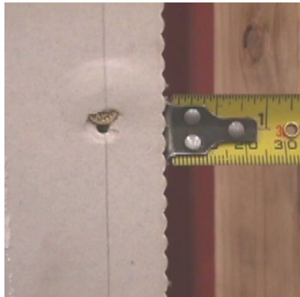
Fig. 5 Typical failure mode of a nail connection between plasterboard and frame in shear. (Note: Tearing of plasterboard and embedment of the nail head within the thickness of the board).
