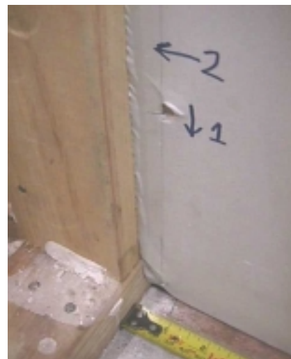
Fig. 6 A photo showing the plasterboard bearing on the corner studs for Wall 1 (as per bottom left corner of Fig. 16).
